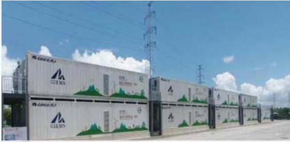
National Biggest 200MWh Smart Microgrid Industry Park
